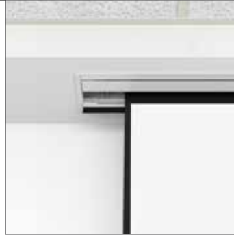
In Ceiling (Open)
